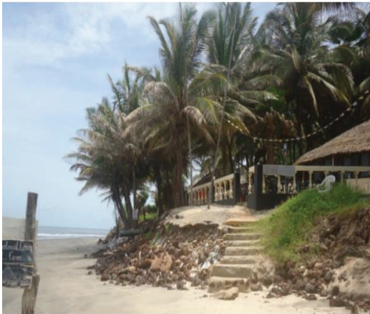
(iii) A Structure at Risk Due to Coastal Erosion
