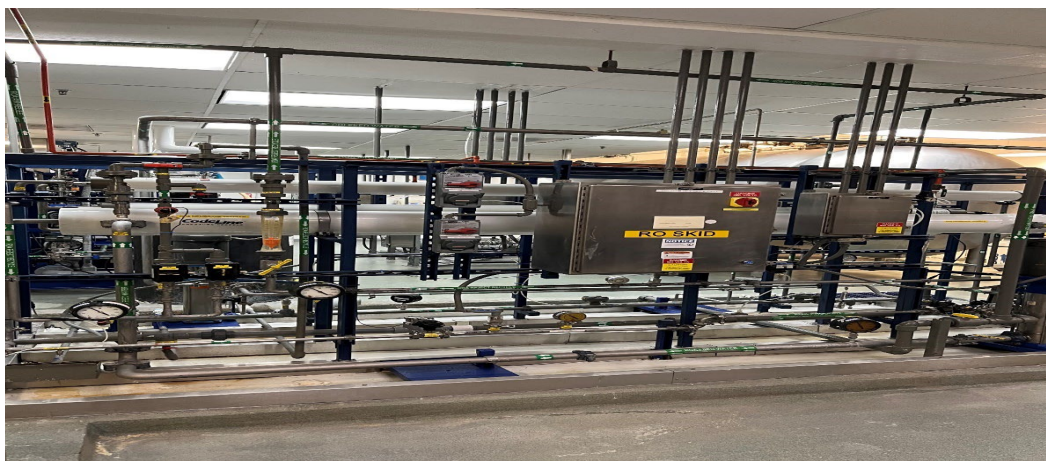
Fig. 5: First pass of membranes (reverse osmosis)
