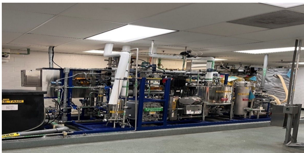
Fig. 2: Smaller scale reverse osmosis system for water purification in manufacturing
