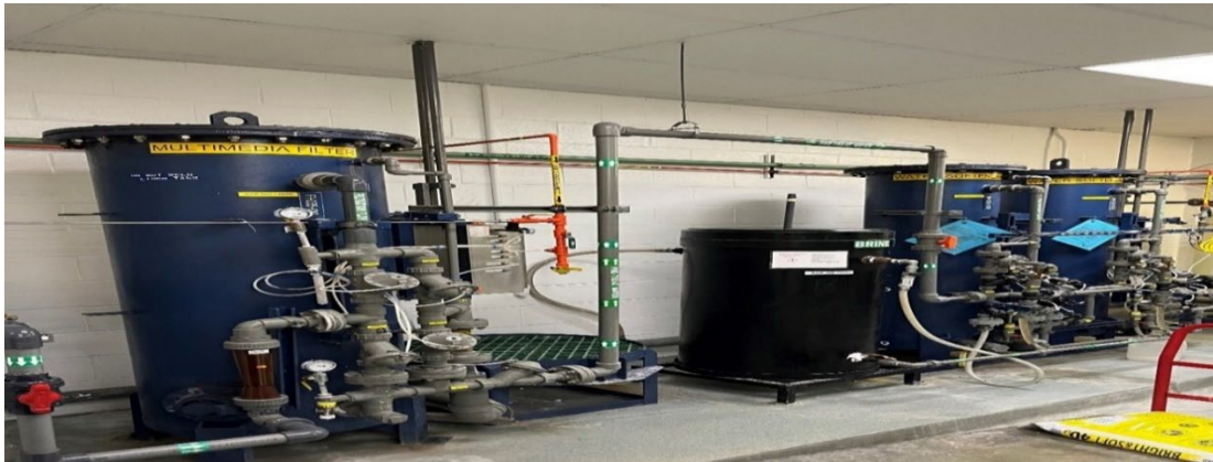
Fig. 3: Multimedia (sand filter) and smoothers
